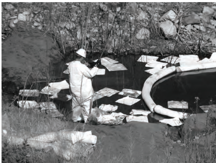
Workers use floatation devices, absorbent pads, and vacuum trucks to remove oil from a creek near the Sespe Condor Sanctuary in Ventura County.
